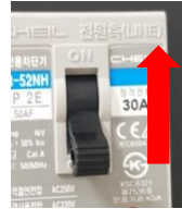
Main Power Switch
